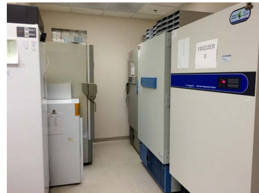
Six -80°C Freezers, One -20°C Freezer and Two 2-8°C Refrigerators
